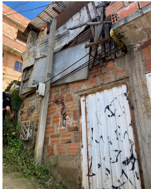
Figure 6: Right. Structural and construction deficiencies. Housing in Ciudad Bolívar. (2022)
