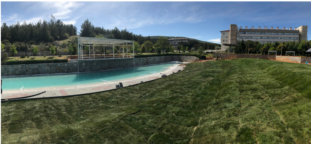
Figure 9: (a and b) Construction phase of the pond on the valley floor, and (c) installation phase of the stage and the grass amphitheatre Source: Authors (2019)
